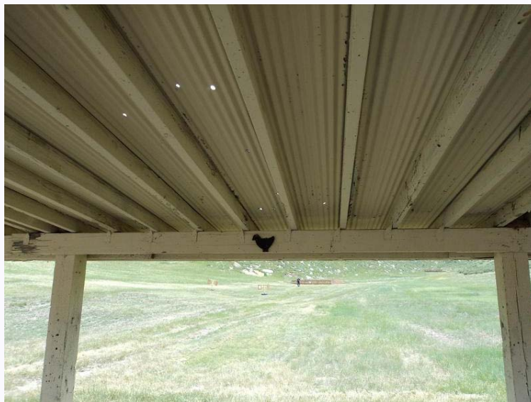
Bullet holes on the roof of the rifle range.
